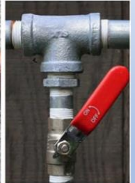
Galvanized Steel & valve
