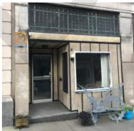
Example of a replacement storefront that is not appropriate.
