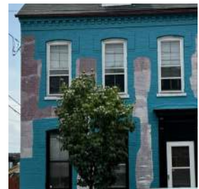
Example of inappropriate use of paint on masonry substrates, as well as inappropriate color choice
