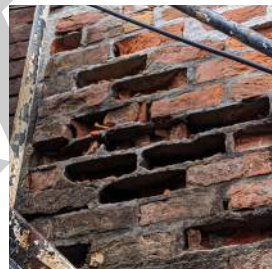
Example of deterioration to masonry caused by inappropriate strength mortar repair
