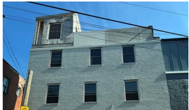
Example of an inappropriate rooftop addition.
