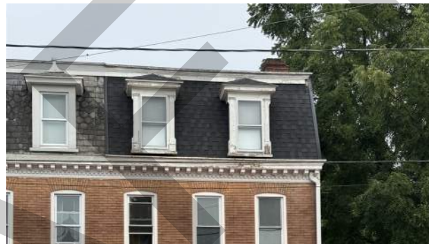
Example of roof inappropriately replaced with asphalt shingle adjacent to historic slate roof
