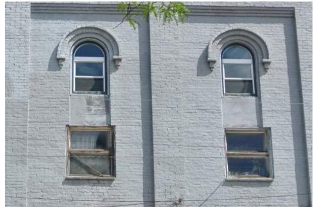
Example of replacement windows that are inappropriate and do not meet the guidelines
