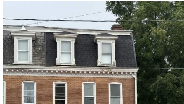
Example of roof inappropriately replaced with asphalt shingle adjacent to historic slate roof
