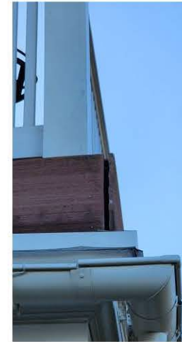
Examples of rotting railing (above) and warped decking (left)
