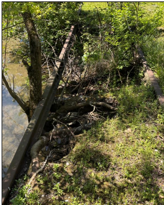
Photo 8 – Rail over eroded bank along Spring Creek, Looking West
